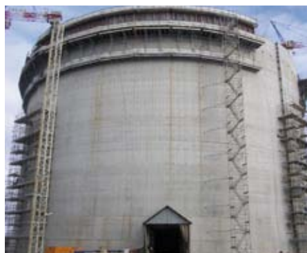
Sakhalin, Russia, 2 tanks of 100,000 m 3
