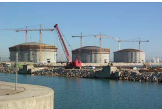
Fos-sur-Mer, France, 3 tanks of 110,000 m 3
